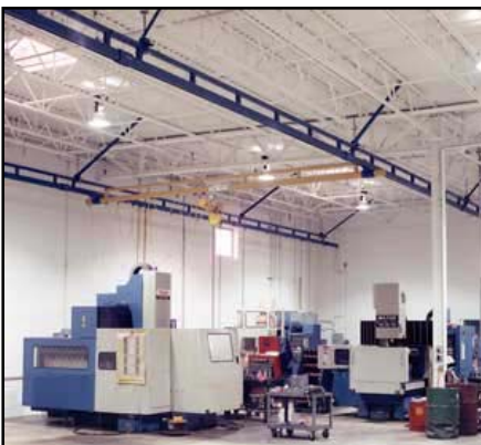
Ceiling Mounted Bridge Crane
